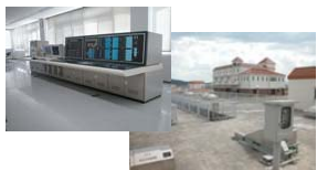
Electric instrumentation systems for water and sewerage
