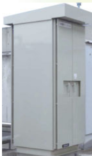
Wind power conditioner*2 installed on a rooftop
