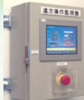
Remote operation and monitoring panel installed in the staff office
