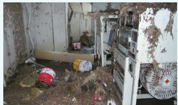
Electric room that had been submerged by the tsunamis
